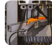
Measurement of leakage current with optional clamp HT96U.
